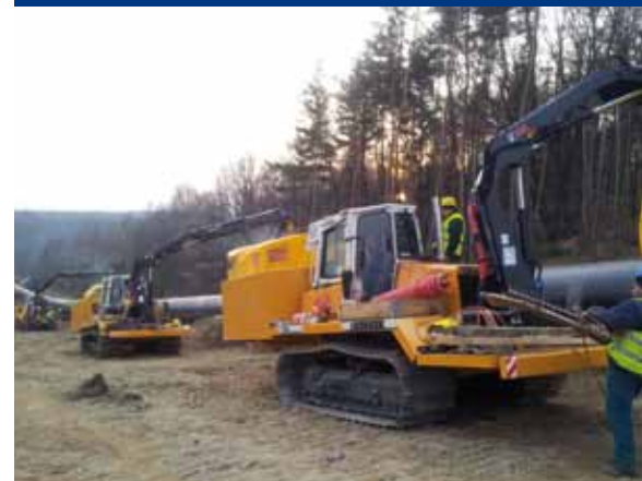
↑ The Kramp workshops installed one additional tandem pump and a specially produced hydraulic system on the Liebherr crane.
